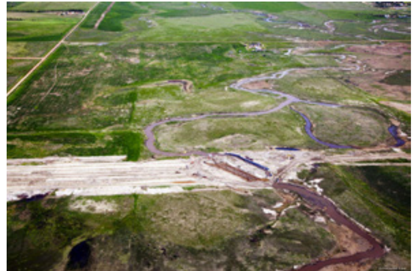
Construction of oilgas pipeline in ND. Photo by the National Parks Conservation Association, 2014.
