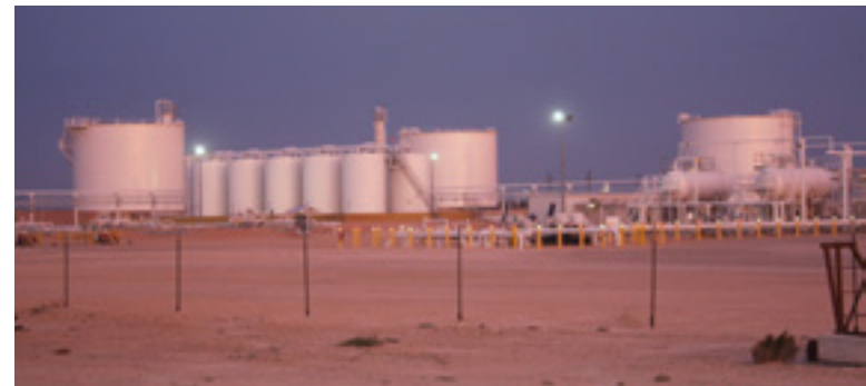
A centralized production facility (CPF). Photo provided by Shell Oil Company.
