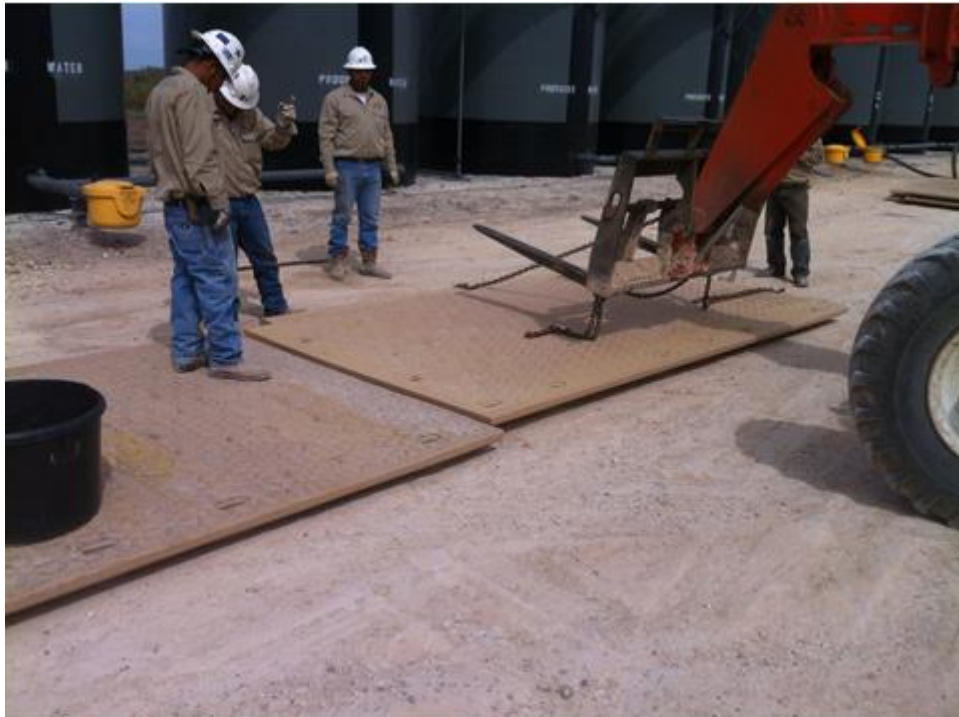
Figure 46. Use of forklift to spot and place mats along proposed road section.
