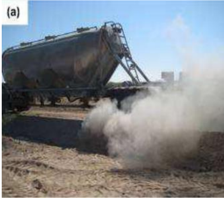
Figure 5. Bulk truck carrying mix for spine road. Dust from blowdown of material after unloading on site.
