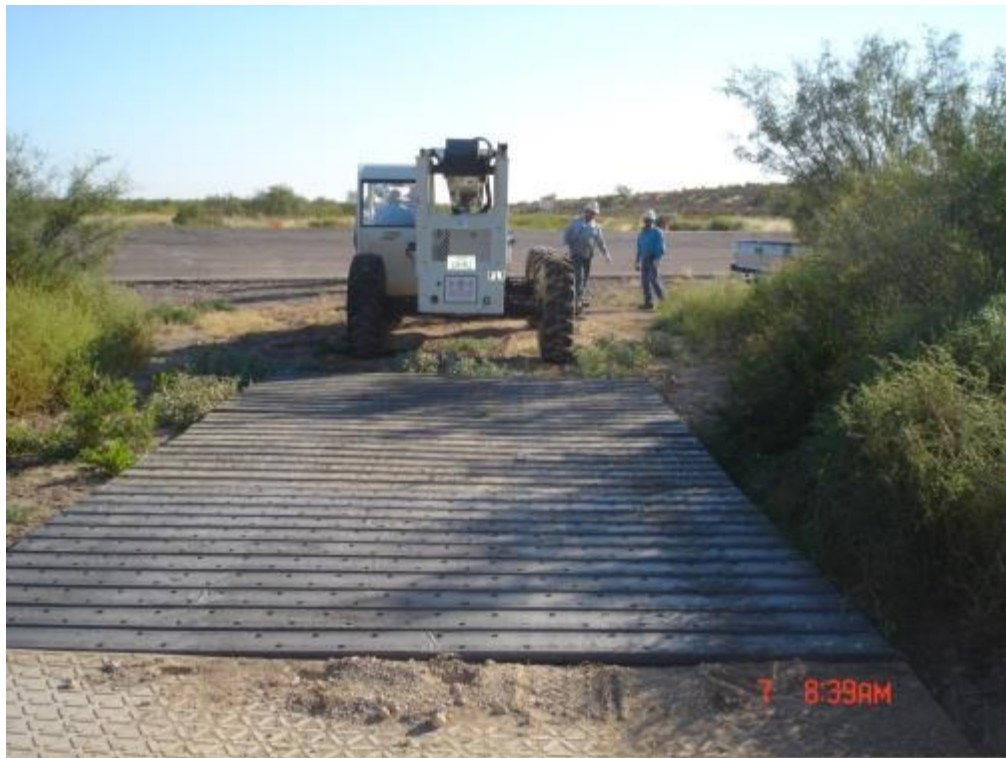
Figure 19. End of installation of Wyoming flat mats, crew ready to begin rollout installation.
