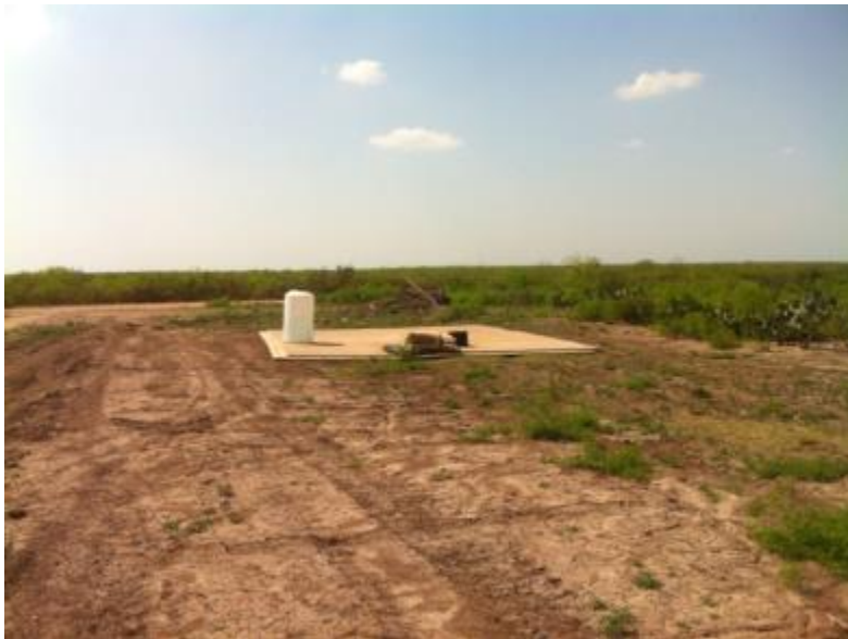
Figure 56. Final layout of pad before equipment move in and setup. Pad on unconsolidated soil not a prepared pad.
