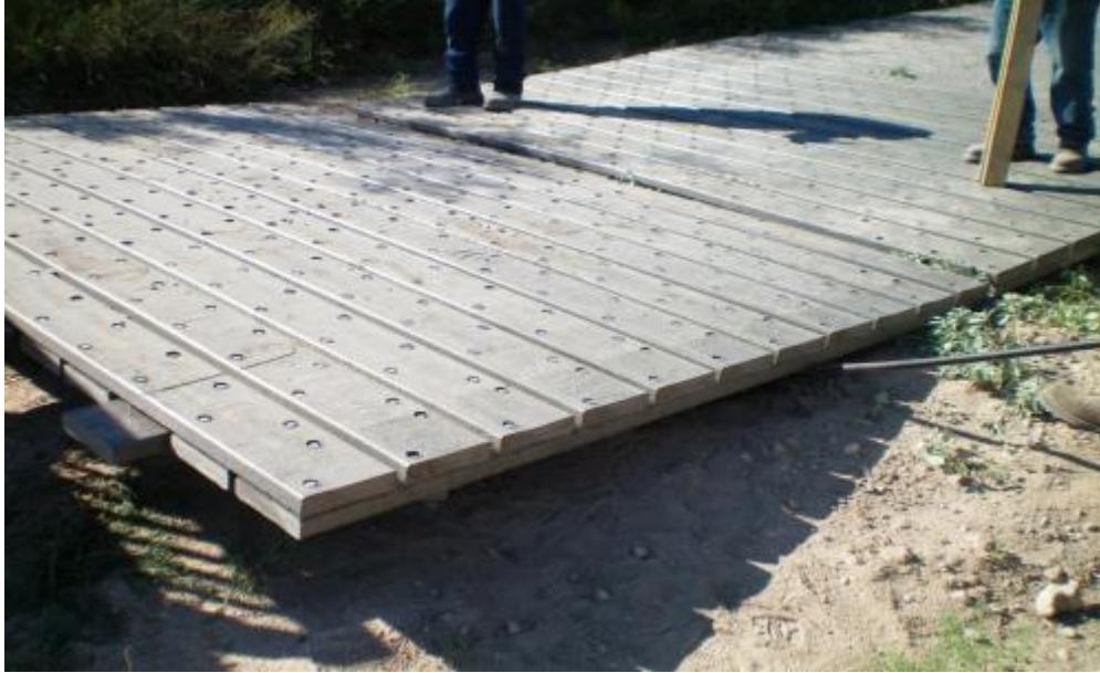
Figure 14. Dipping of front edge of Wyoming Flat panels to match new panel to previous installed panel before final layout of unit.
