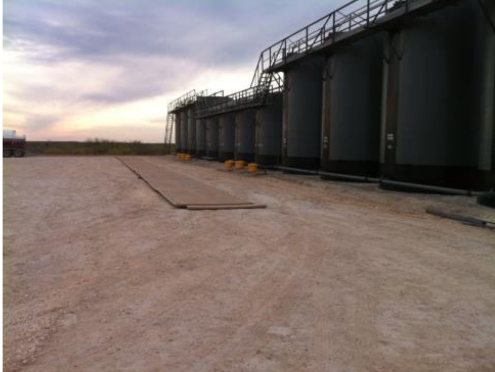
Figure 47. Completion of first row of roadbed. Note road not wide enough for large vehicle and overhang on left side of panel could be a problem.
