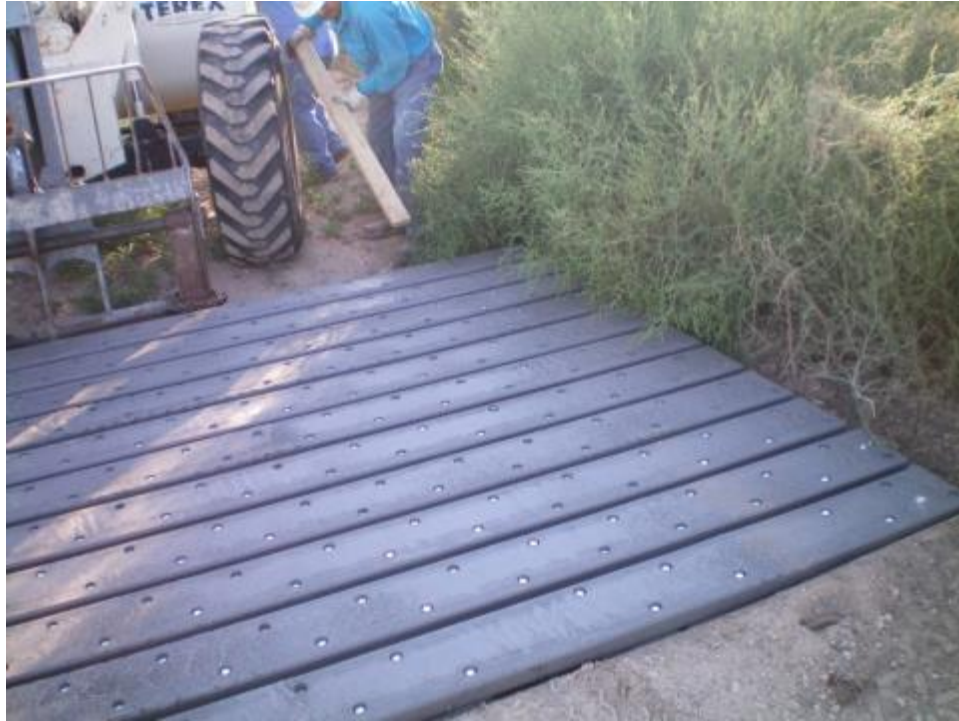
Figure 12. Wedging of Wyoming Panel to match Newark Mat. Newark mat set with an overlap on this side of panel to match the Wyoming panel setup.
