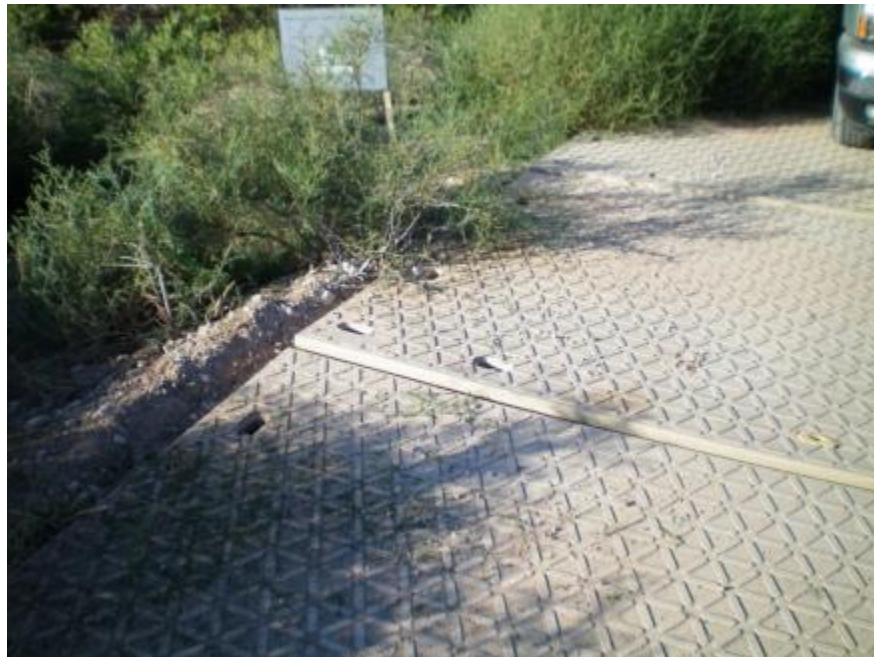
Figure 38. Outside edge of Newpark mats indicate buckling potentially caused by lack of keylock to connect panels.
