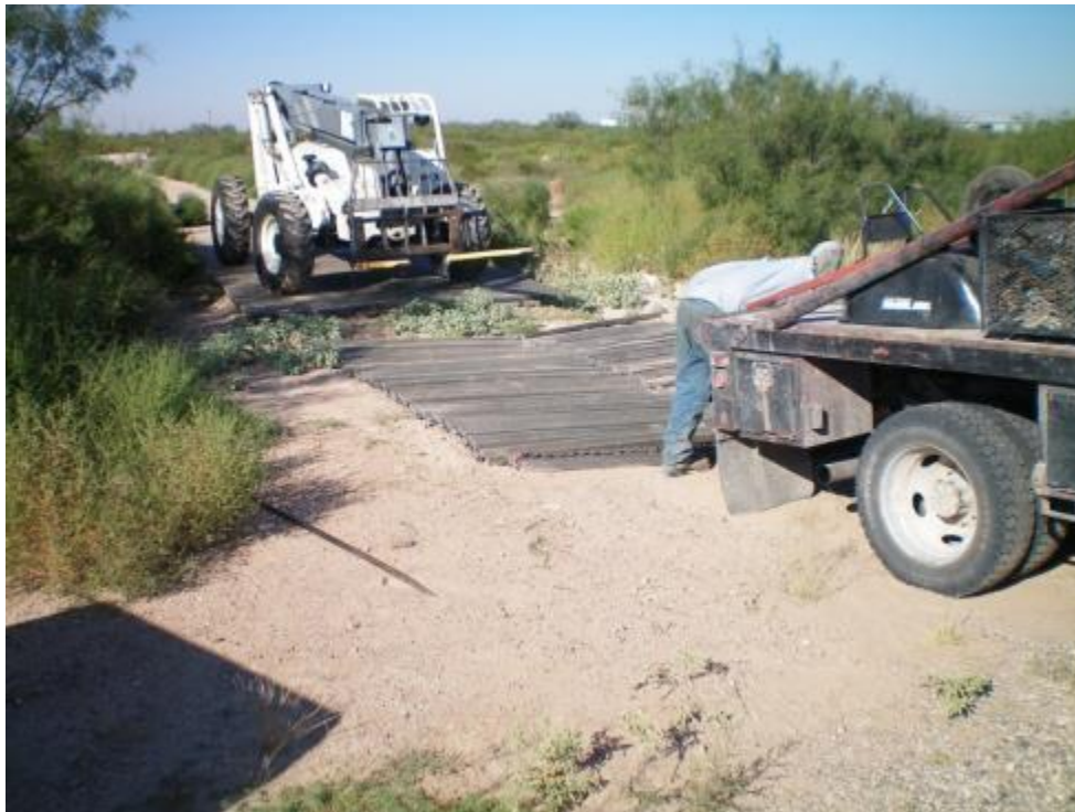
Figure 23. Laydown and drag out of first Wyoming rollout panel. Requires both the forklift and roustabout truck for placement.
