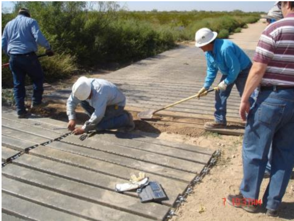
Figure 29. Backfill of transition point between fixed panel and rollout mat using broken sections as grade transition between units.
