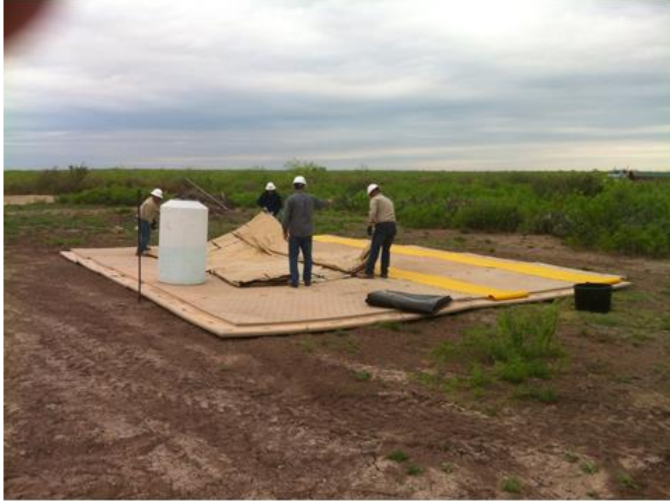
Figure 57. Layout of containment on pad to prevent leakage. All equipment of field trial will be on a pad made from some type of artificial material.
