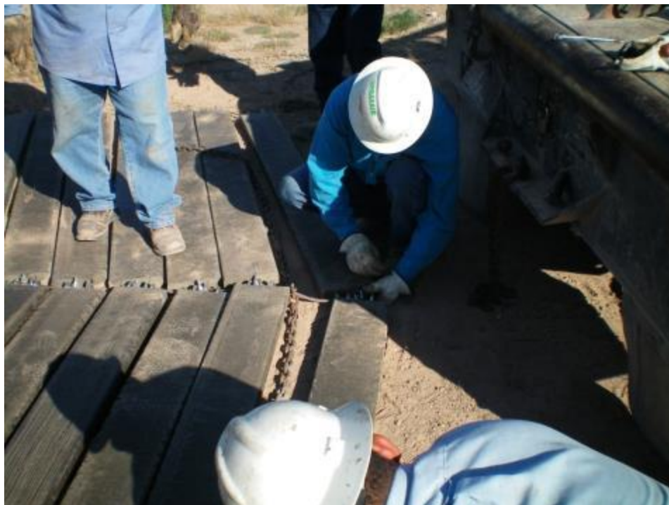
Figure 27. Removal and replacement of broken section of mat during installation. Required removal of locking clamps on each end of board to be removed.
