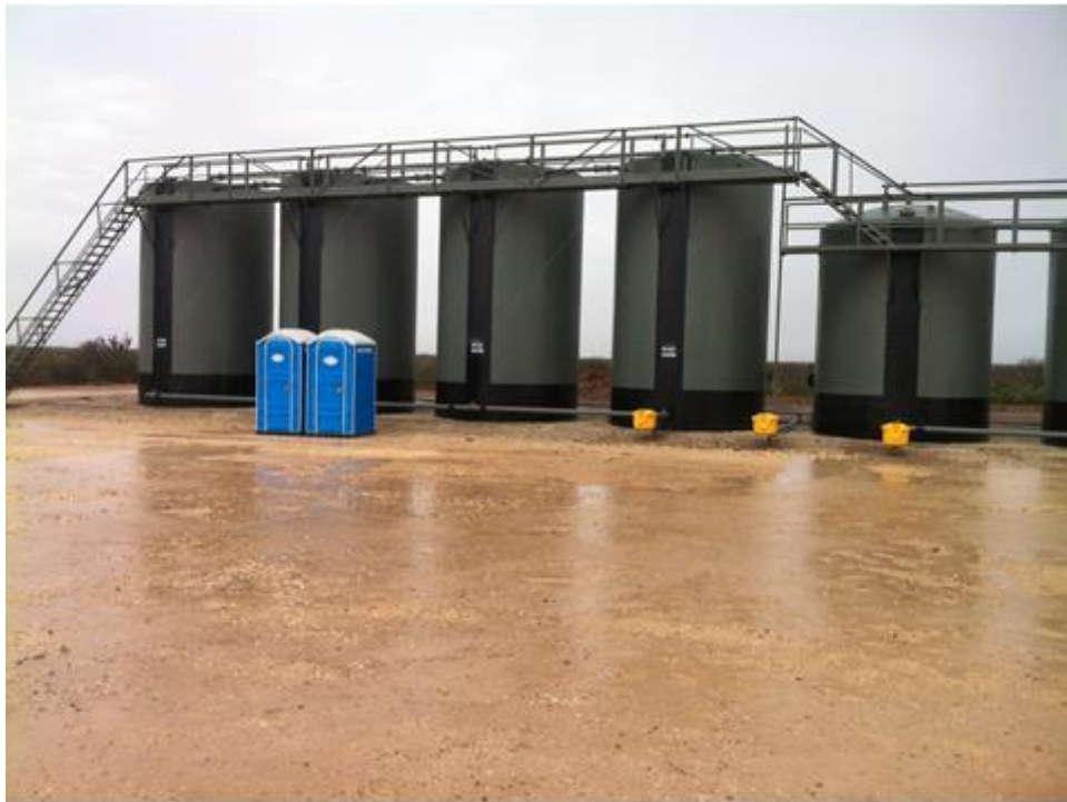
Figure 44. Test Site in Eagleford Shale area, note muddy location with soft clay content of caliche.
