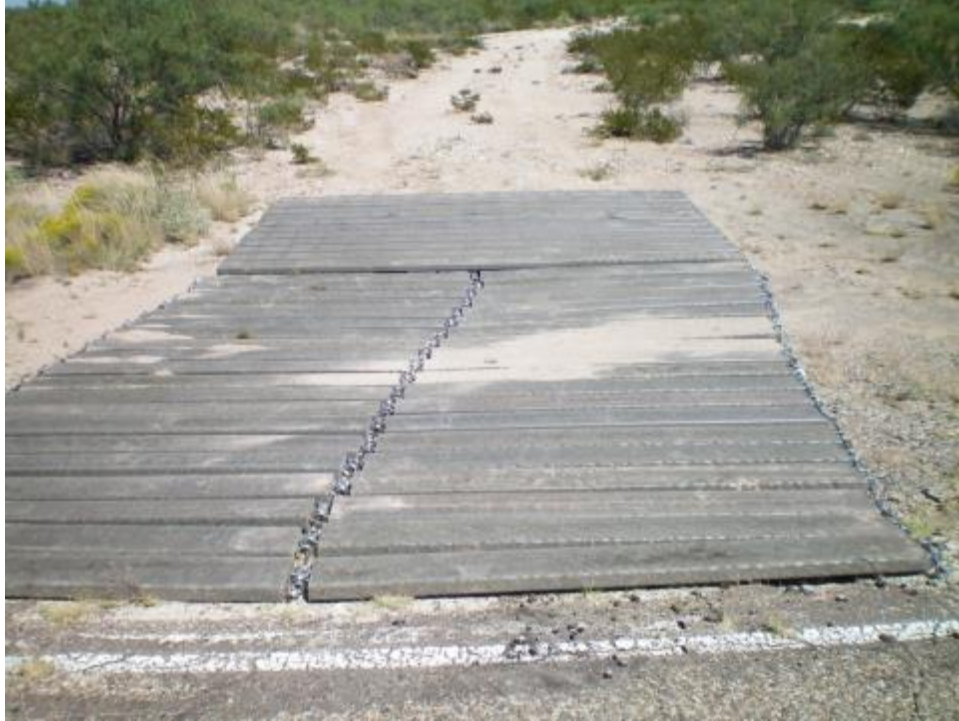
Figure 35. Final layout on Wyoming and rollout panels on exit from field road to paved street. Note nonlinearity of roadway with use of the rollout panels.
