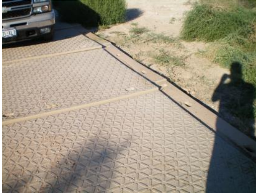
Figure 37. Note washboard buckling due to lack of connection between mats. Only two pins/locks were used per connection. The panel allows for a total of 5 per connection.
