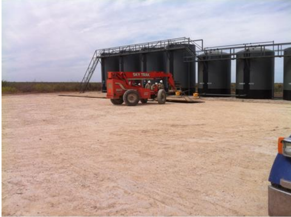
Figure 45. Initial setup and layout of road panels before containment built for tank battery.
