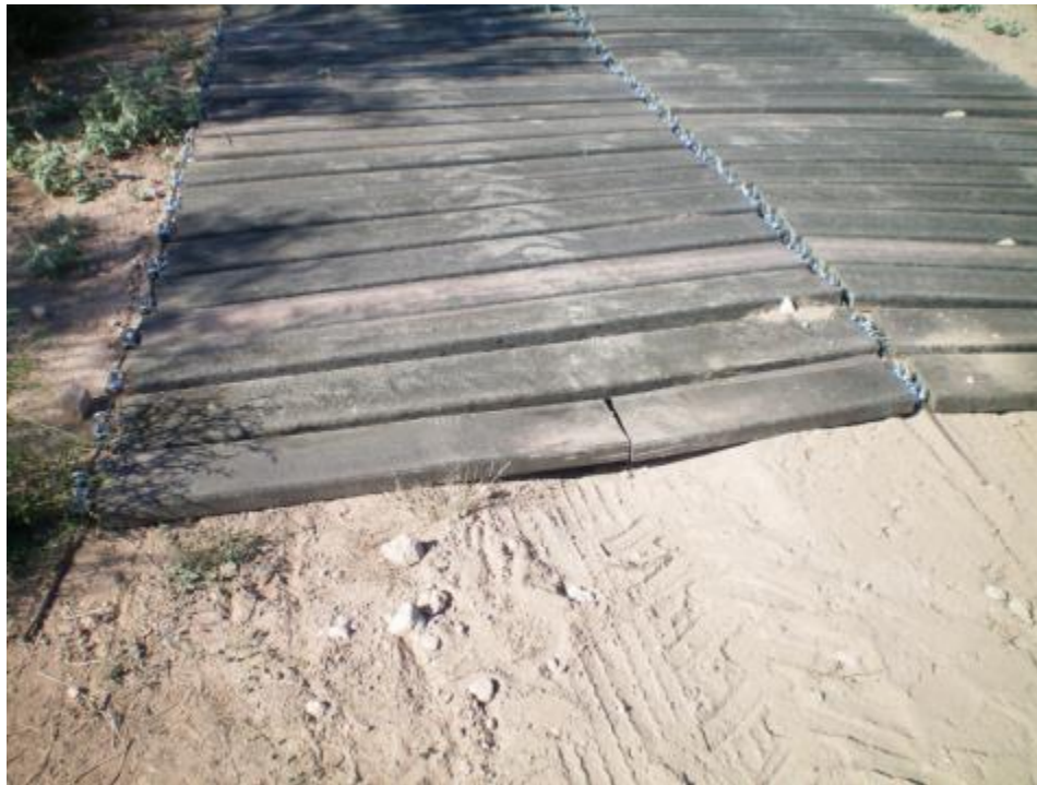
Figure 25. Note broken board section at end of panel. Cause of break can be seen by tire print on panel and the washout below the break in the board. The design of these mats gives strength in only one direction. To obtain maximum strength panels need bi-directional construction to prevent failure.
