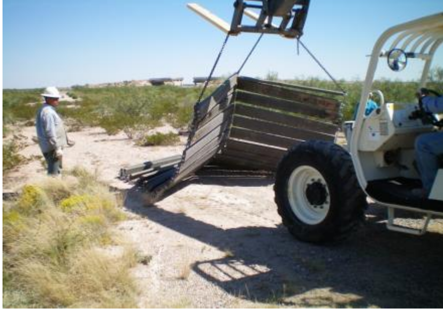
Figure 31. New Approach to installation of rollout panels. This required the chaining of the panels to the forklift to allow a vertical pickup with the panel hanging below the forks of the unit.
