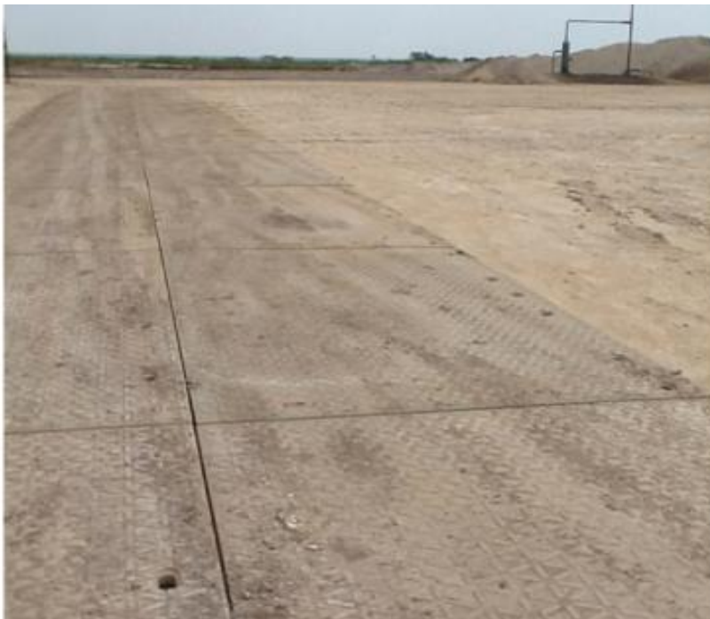
Figure 52. Final installation of road mats after construction of containment. Note the traffic patterns on the mats showing the drive up on to the road as well as the departure from road after loading.
