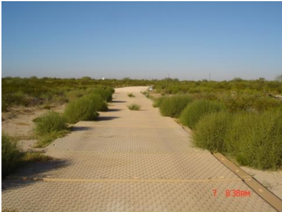
Figure 36. View back on Newpark panels installed earlier in project. Note the growth of tumbleweeds along edge of road and at unions between panels.
