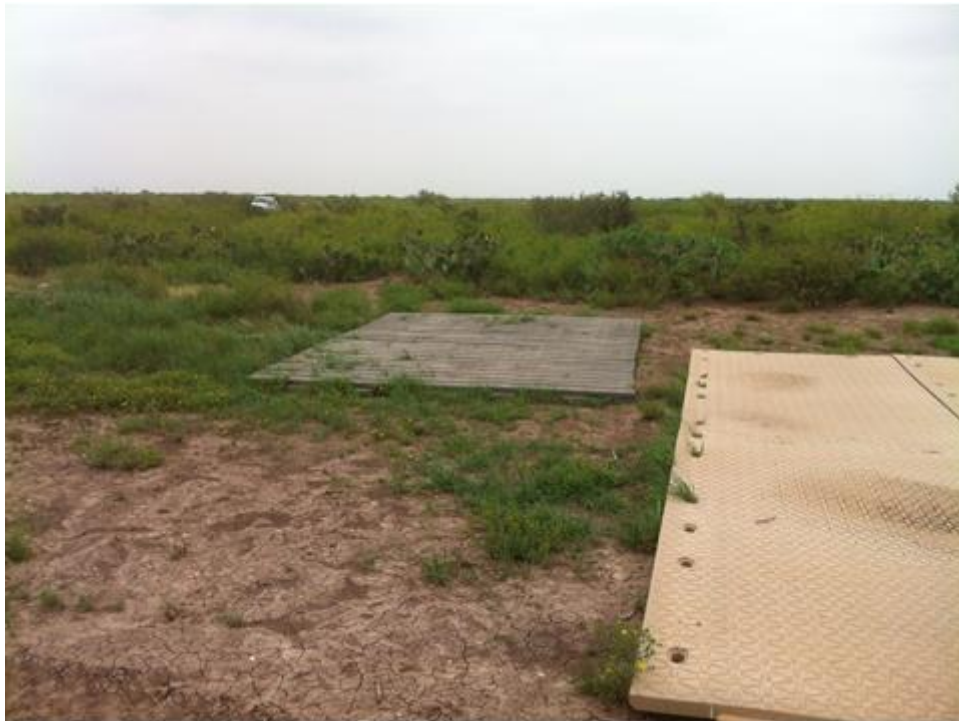
Figure 58. A secondary pad was made using the Wyoming mats for the generator. The size of the mat matched the size of the containment for the unit to be used.
