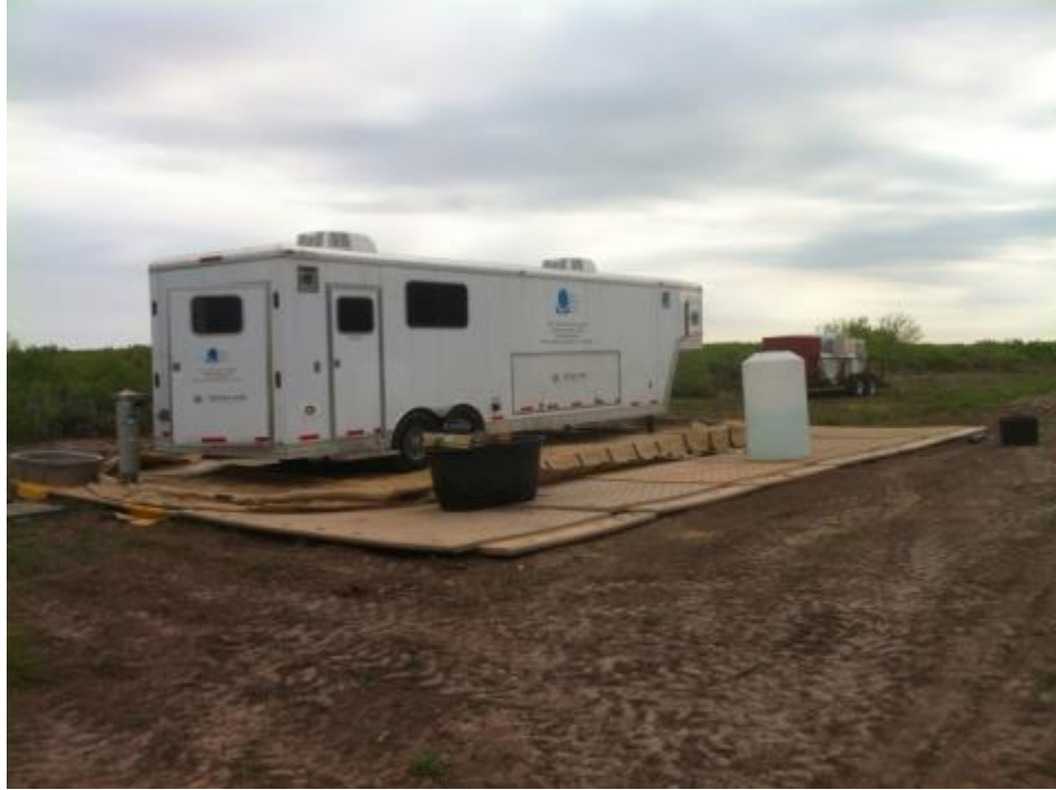
Figure 59. Final install of field trial equipment on pad using Newpark mats. Note we used a total of 10 mats for the pad.
