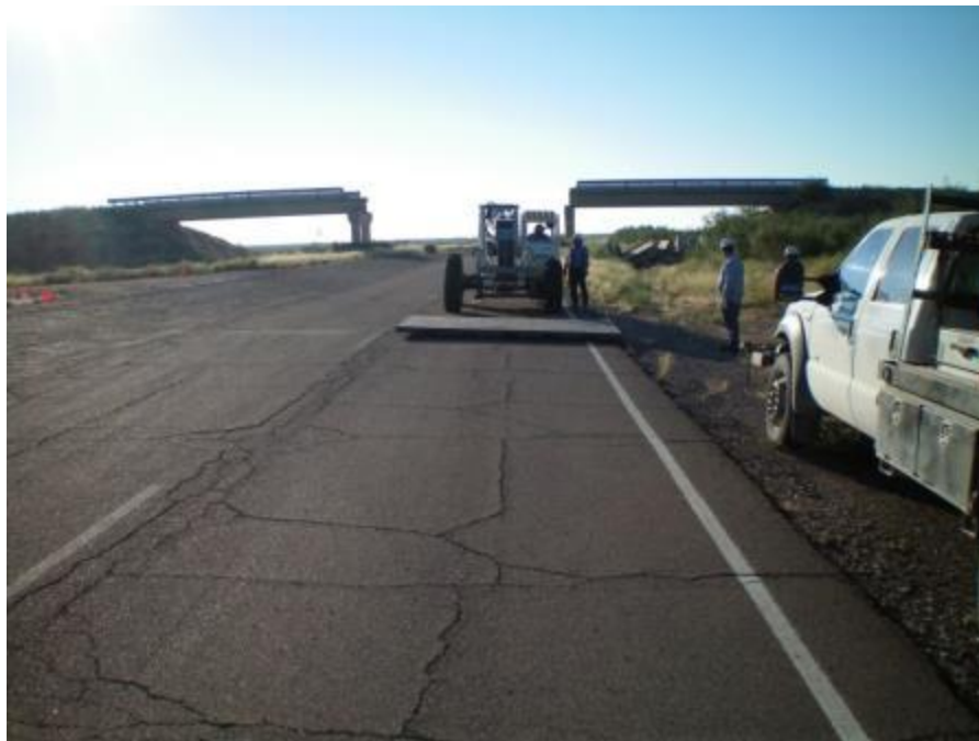
Figure 11. Movement of fixed Wyoming panels to road-site at bypass for overpass out of service.
