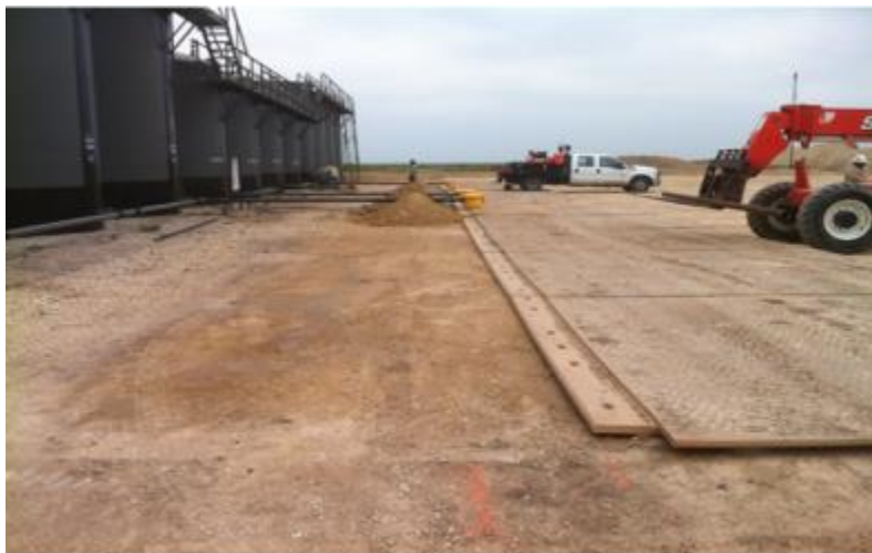
Figure 50. When ready to install the containment the road section needed to be moved for the installation. In this case two backhoes were used to drag the section approximately 8 feet to allow for containment.
