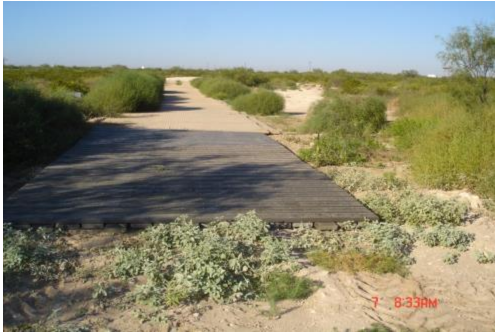
Figure 18. Back view of road sections note straight line of road. Special care is required to prevent a lateral slippage during installation that can cause problems later depending on length of road.
