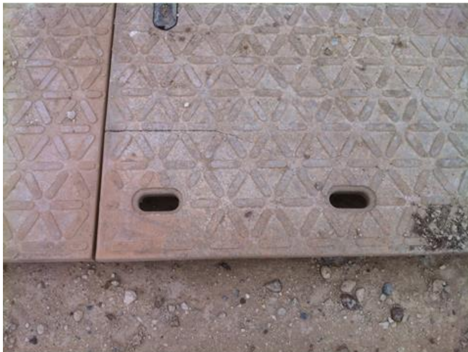
Figure 60. On several mats stress cracks occur at the union point between the upper and lower section of each mat.
