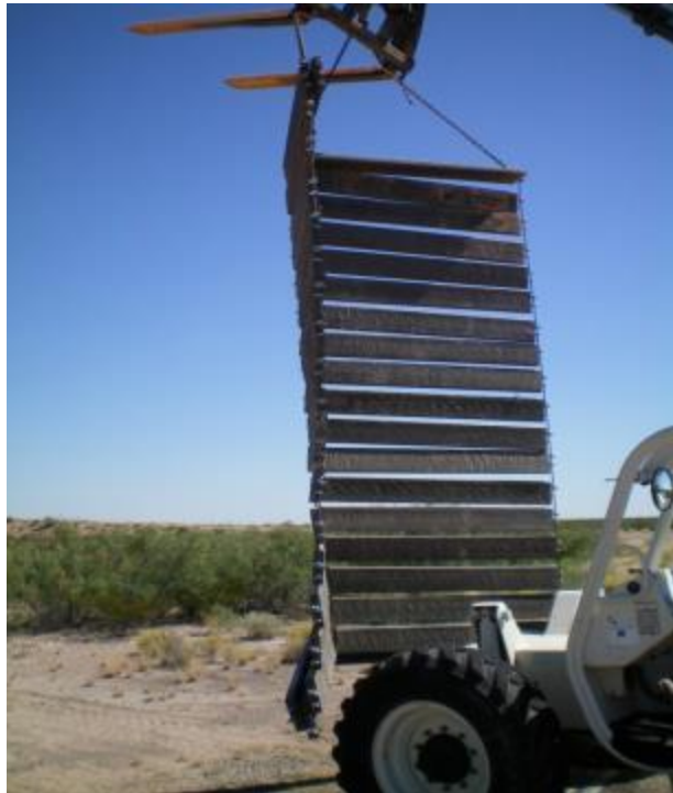
Figure 32. Extended View of rollout panel after pickup using new approach for installation. Panel is pivoted in middle but addition of steel stringer or section with chains would remove it and allow a straight hang of the panel before laydown.
