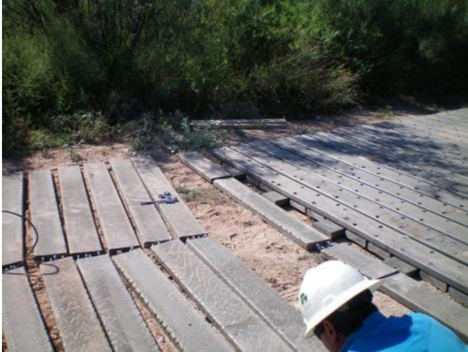
Figure 28. Placement of broken sections at union between fixed mat and rollout mat during installation. Note that vertical transition is attained using broken board sections as lift points on the mat.
