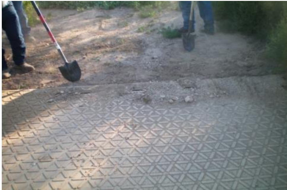
Figure 10. Cleanout of dirt and weeds at transition between Newpark and Wyoming mats.
