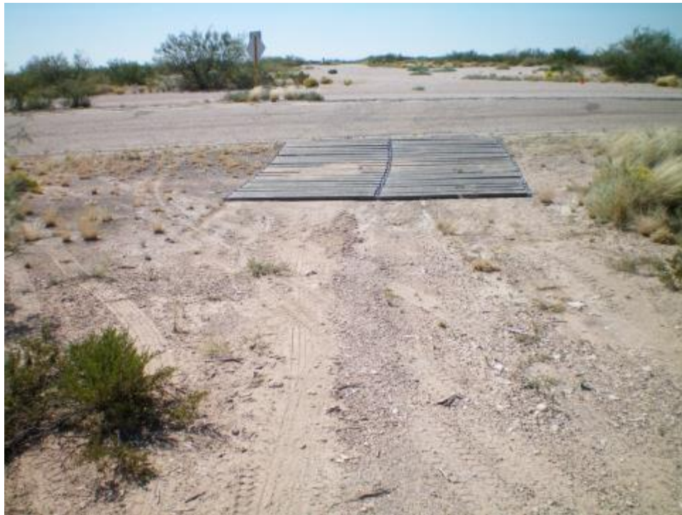
Figure 34. View of Rollout panels after placement. Note twist or nonlinear direction of panel as installed.
