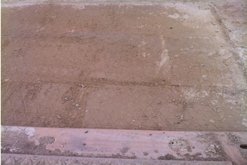
Figure 51. This indicates the amount of embedment of the mat into the caliche base on the location. The mat tends to imbed to some extent depending on the strength and integrity of the base material.
