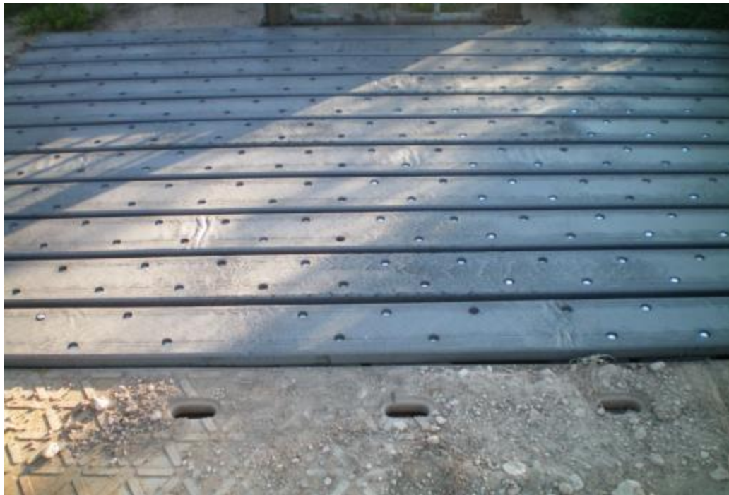
Figure 13. Transition between Newark and Wyoming panels in final layout of Pecos road section. Thickness of both type of panels similar and did not require major movement of soil to match panels.
