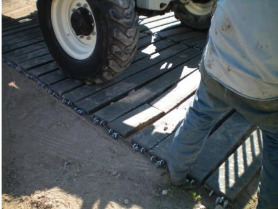
Figure 24. Note Break in interior board of Wyoming Rollout panel.
